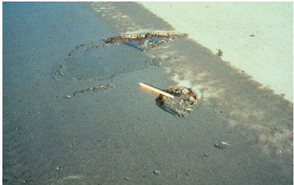
Figure 2.2.20 Spalling on a Concrete Deck
