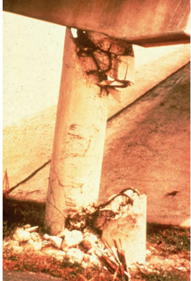
Figure 2.2.23 Concrete Column Collision Damage
