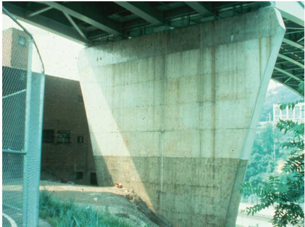
Figure 2.2.28 Anti-Graffiti Coating on Lower Area of Bridge Piers
