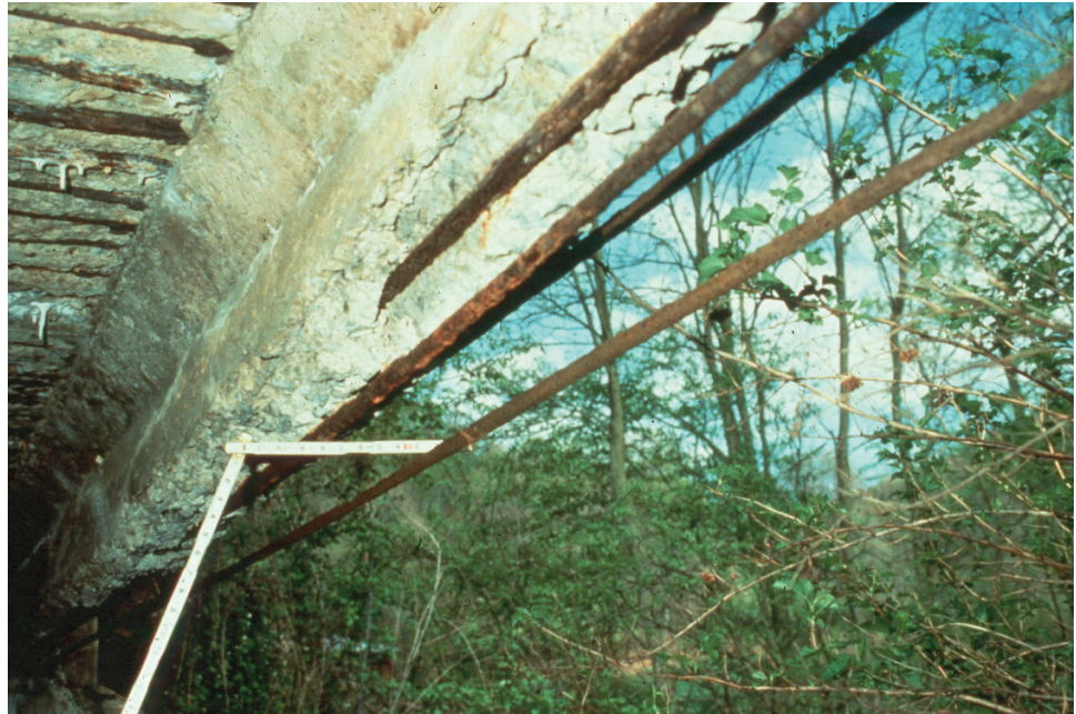
Figure 2.2.26 Loss of Bond: Concrete / Corroded Reinforcing Bar
