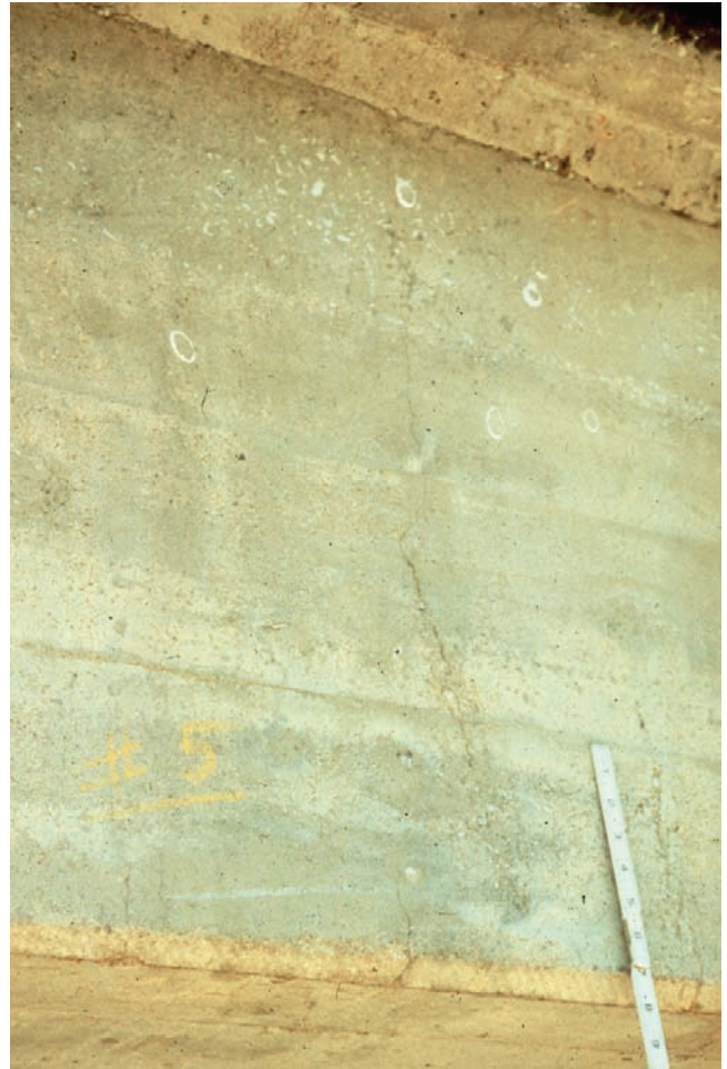
Figure 2.2.7 Flexural Crack on a Tee Beam
