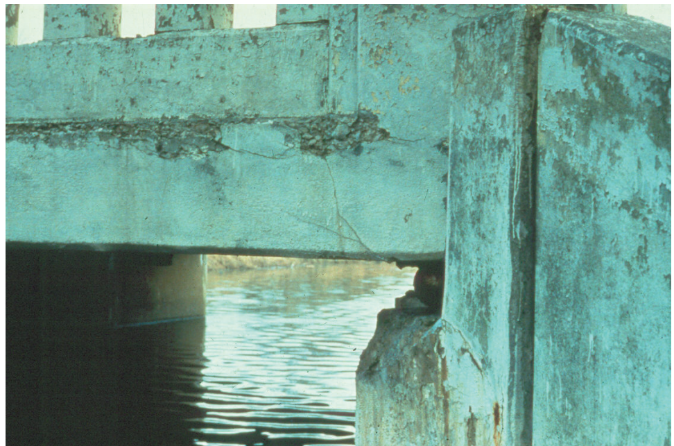
Figure 2.2.8 Shear Crack on a Slab Beam
